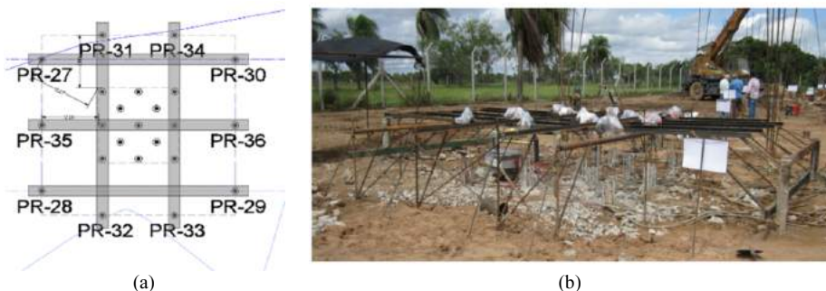
Figure 7. (a) General arrangement of at the test, showing reaction piles and beams; (b) Frame for recording pile movements Phase 1 test on Piles E2 - E14.
