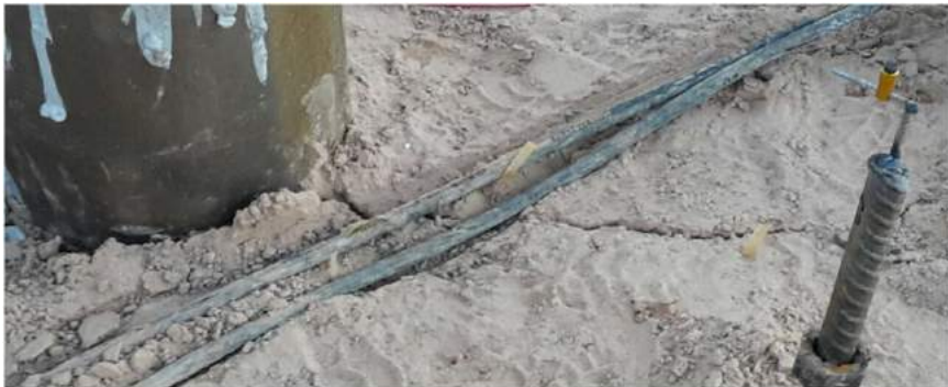
Figure 14. Photographs of cracks in ground surface stretching from one pile toward the next along the side of the group.
